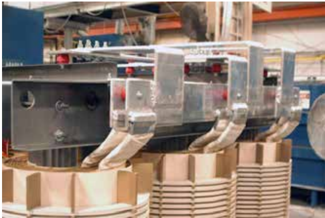
Figure 5. MIG welded leads to AL bus.
