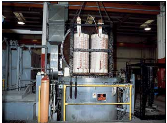
Figure 9. Coils after VPI process ready for baking in the oven.
