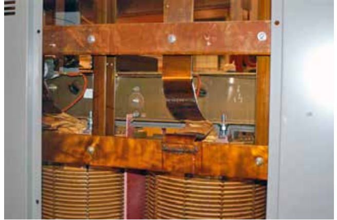
Figure 7. Brazed copper LV lead to Cu bus.
