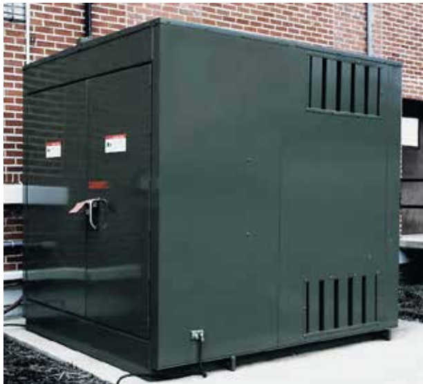
Federal Pacific Pad-Mounted Transformer.
