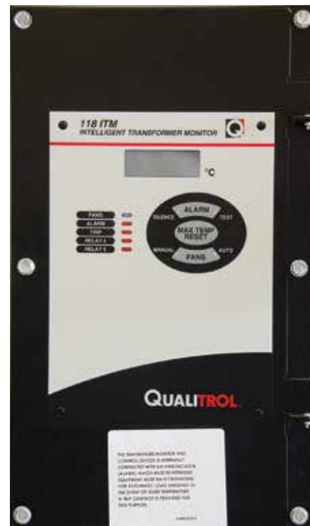
Federal Pacific's preferred temperature monitoring device.
