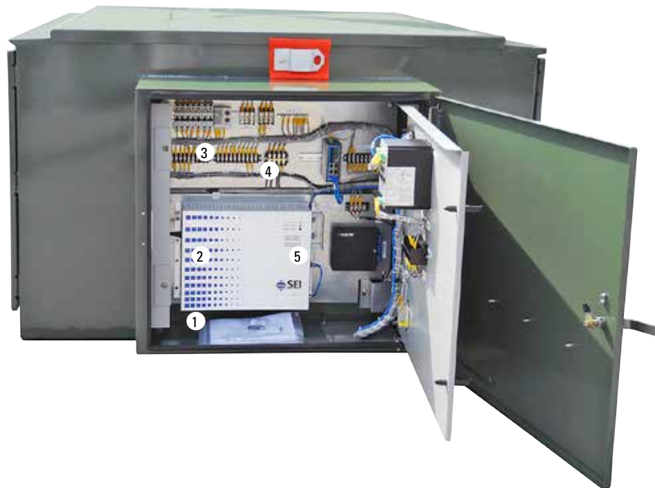
Figure 6. Opening the hinged panel provides access to the remaining low-voltage components. Included are (1) the instructions and drawings on the bottom plate; (2) an SEI UPS Power Supply; (3) secondary circuit breakers, thermostat and heater (not visible); (4) an Ethernet switch; (5) a Black Box patch panel, and all the associated terminal blocks.
