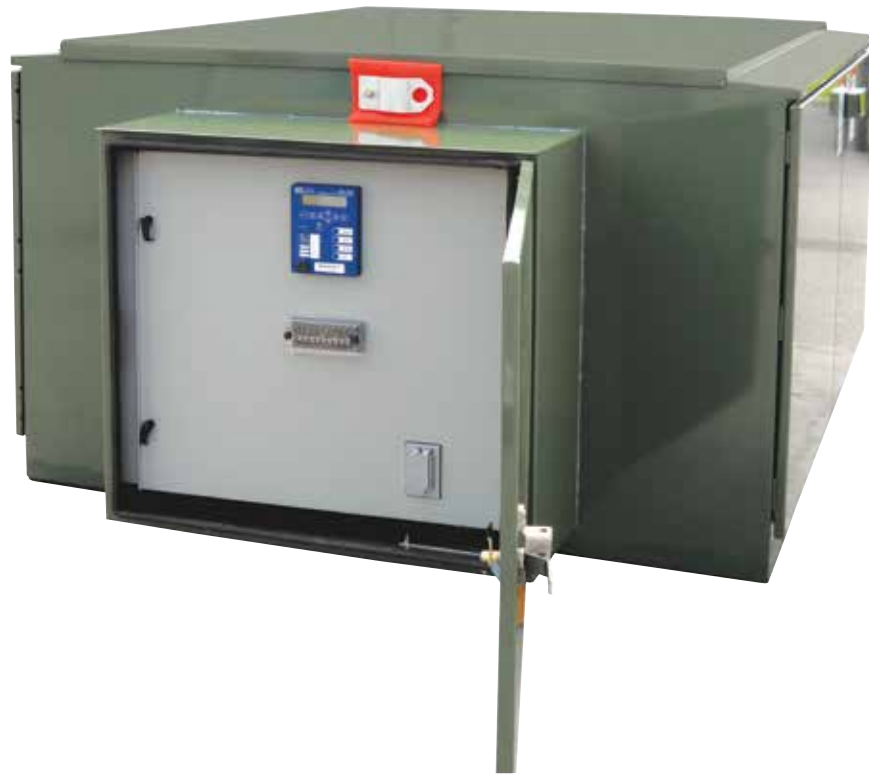
Figure 5. The SEL-735 Power-Monitoring relay is panel mounted on a hinged steel plate, which also provides the mounting surface for the test switches (in center of panel) and the 120vac outlet (at lower right on panel).
