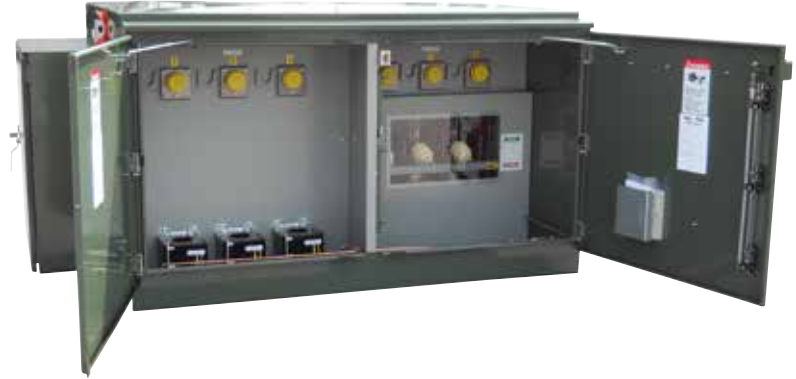
Figure 2. Open door view shows incoming termination compartment at right with incoming load-interrupter switch visible behind viewing window. Outgoing termination compartment is at left and includes sensing CTs to measure and confirm load current and provide that input to the power monitoring relay. The voltage transformers are mounted in the interior of the switchgear.
