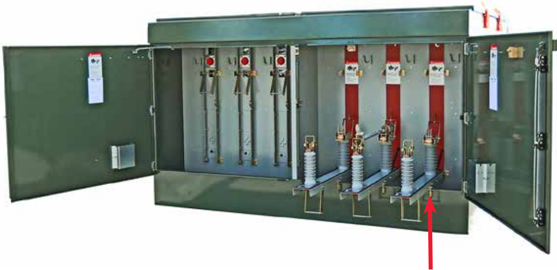
Figure 6. Fuse panels are shown open in one fuse compartment, revealing the typical shutter barrier that closes over the opening to maintain isolation of the interior high-voltage compartment. Fuse assembly is shown installed in center phase. Note that fuse panels are locked down using the locking bracket that secures the fuse panel to the door-opening flange (at arrow).
