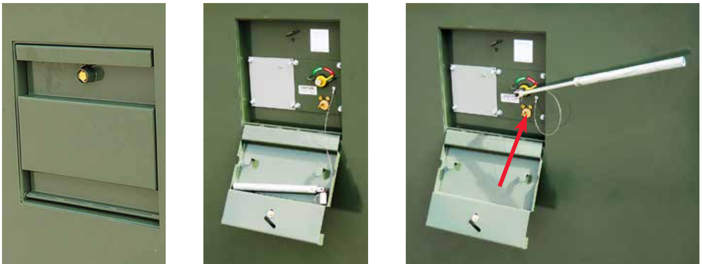
Figure 8. The switch-operating handle and its storage pocket are pictured above. The pocket and cover (and its hinge) are of stainless steel. The cover is secured closed using a pentahead bolt and is also padlockable. The handle, which is extendable, is held in place by two clips on the back of the cover when the cover is raised. The handle pocket includes a one-line diagram, a green (open) and (red) closed position indicator with a yellow lever pointing to show the actual switch position. A key interlock (at arrow) is provided and is held captive when the switch is closed. When the switch is opened, the key can be turned and removed, allowing it to be inserted in the corresponding key interlock on the access doors to fuse compartments, so they can be opened. It is this sequence that insures that the circuit is open on the incoming side, de-energizing the fuses (unless backfeeds exists, which must be confirmed by checking for the presence of voltage) before access is obtained to the fuses.
