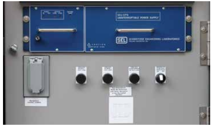
Figure 7. The Federal Pacific automatic-transfer scheme includes a UPS (at top in photo), test pushbuttons to simulate loss of source voltage and over-current lockout to allow verification of the functionality of the transfer scheme, and a duplex outlet for connection of a laptop computer. Also see Figure 6.
