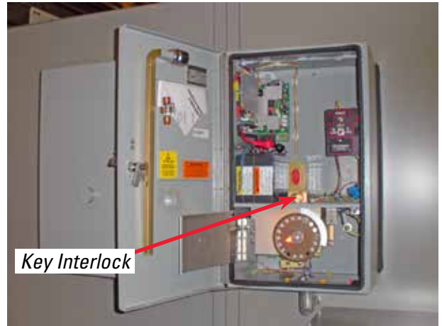
Figure 5. The Fast-Trip Motor Operator is illustrated above with the interlocked cover over the motor shown closed in the top photo above and with the cover open in the bottom photo above. As the motor rotates at high speed, if the cover is open motor operation is suspended. A separate key interlock (see arrow in photo) can be provided to block operation of the motor operator for other specific requirements, such as requiring that all switches be open before allowing access to fuses.
