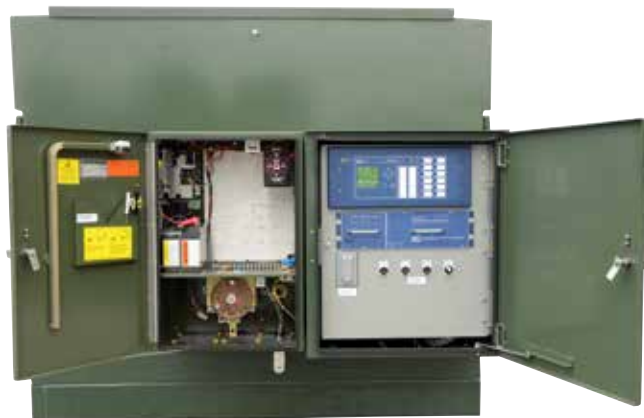
Figure 2 – In this view, the doors of the low-voltage cabinets are open, showing the standard run-and-trip motor operator in the cabinet to the left, and the control cabinet, featuring the SEL-451 relay, in the cabinet to the right. The control cabinet is shown in detail in Figure 6.
