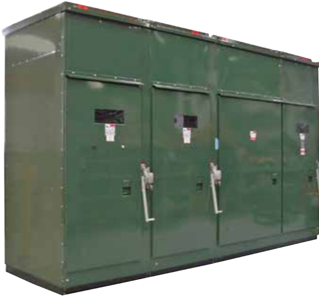
Figure 1. A 4-bay, 25kV, outdoor lineup of Federal Pacific Metal-Enclosed Switchgear provides primary power with utility metering to two connected lateral load-feeder circuits. See one-line diagram on page 5.
