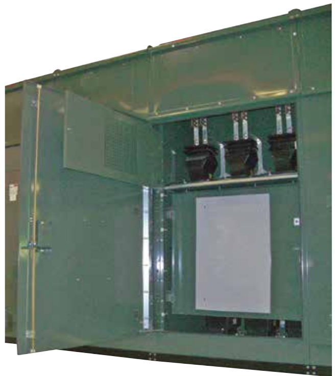
Figure 3. Open door view of metering bay showing (at left) a hinged protective screen at top section over current transformers and a hinged- panel with a plywood section for meters and controls to be installed by the utility. The perforated screen allows viewing the CTs without opening the screen. With the screen open (in photo at right), the revenue metering, outdoor-style, current transformers are completely visible for closer inspection.
