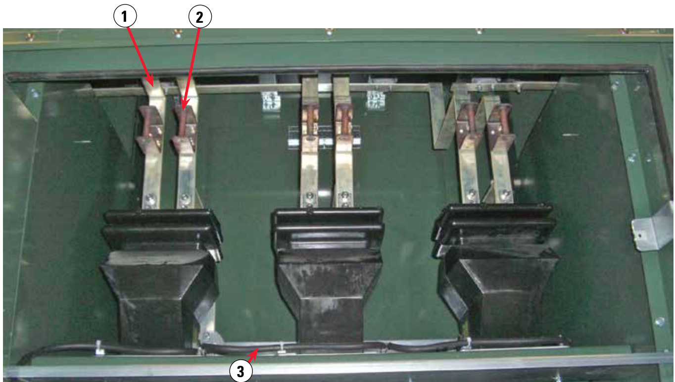
Figure 4. Close up view of compartment containing current transformers shows (1) bus interconnections (2), grounding provisions on each CT terminal, and (3) interconnecting ground cable that runs to compartment ground pad. CT secondary wiring is isolated in conduit and connects to a terminal block with shorting pins, which is located on the side wall of the enclosure. CTs were provided by the customer and installed and wired by Federal Pacific.
