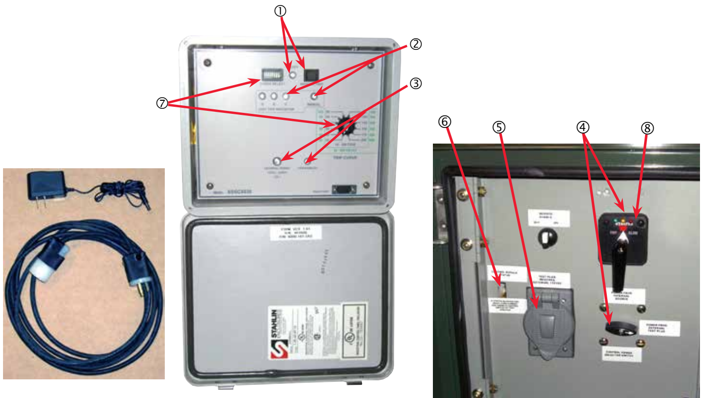
Figure 3. Faceplate of Self-Powered Relay is at center and Control Panel is at right and both are inside the Low-Voltage Compartment. A ten-foot extension cord (at bottom in left photo) is provided for connection of an external 120vac control-power source and a 120 vac/12v dc power cord (at top in left photo) is provided for control power to the self-powered relay.
