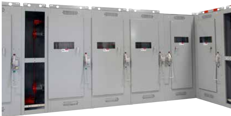
Figure 8. The five (5) feeder bays on the right side of the switchgear assembly are pictured at left. Doors of feeder bays include mechanical interlocks to prevent opening the door until the switch is open. With the doors open, access is possible to change fuses. While the door is open, the switch cannot be operated. Viewing window in each door allows inspection of the interior without requiring that the door be opened
