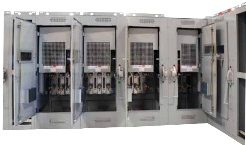
Figure 9. The photo at left shows an open door view of four (4) of the feeder bays on the right side of the bus-tie switch. Perforated steel screens over switches of feeder bays limit exposure to energized bus at the top of the bay when the switch is open and access to the interior is necessary, such as to change fuses.
