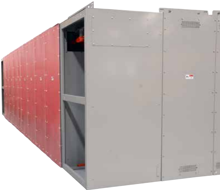
Figure 12. Extending across the entire rear of the switchgear assembly are full-height sheets of GPO-3 grade red fiberglass. These insulating sheets, installed with non-metallic hardware, provide isolation of the metal switchgear surfaces from adjacent energized components that are located in the vault where the equipment is installed.
