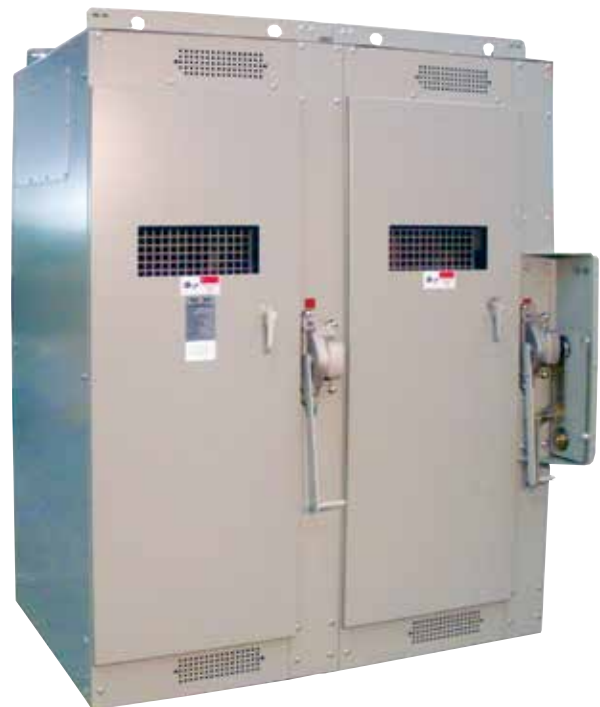
Figure 14. Metal-enclosed switchgear (and pad-mounted Switchgear not pictured) is shown equipped with a Federal Pacific portable remote operating mechanism on the bay at right to allow operation from a distance of up to 50 feet using compressed air or CO 2 .
