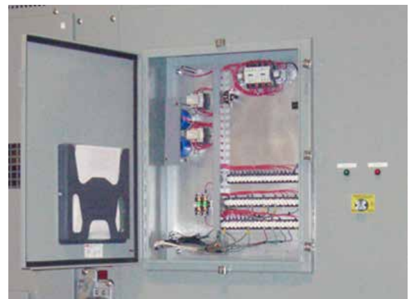
Figure 4. Pictured above is Bay 3, which includes the VBT vacuum interrupter switch for frequent sustained switching of the load circuit. Inset at top (on right above) shows dual, hinged screens allowing separate access to the vacuum interrupter (at bottom in photo at left) and to VTs and CTs (at top in the photo at left). Inset at bottom (on right above) is a view of the interior of the low-voltage compartment mounted in the Bay 3 compartment door and containing the control circuit for the vacuum interrupter; the green/red position indicating lamps for the vacuum interrupter; and the voltage indicator with multiple color-coded LED-type indicating lamps to show presence/absence of voltage on each phase and ground.
