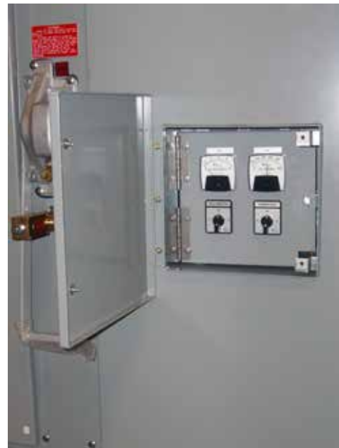
Figure 3. Pictured above is Bay 2, which includes the incoming switch for the alternate (backup) source. Insets show (at top) screen over the switch that is encountered when the enclosure door is opened and (at bottom) the analog voltmeter and ammeter with selector switch, allowing a real-time verification of the condition of the incoming power source. Bay 1, which includes the incoming switch for the preferred (normal) source is similar.
