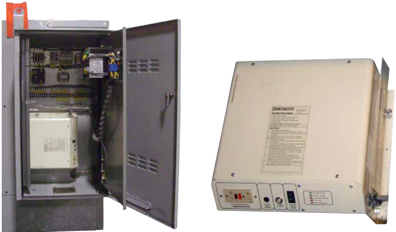
Figure 5. An inverter capable of utilizing a 48vdc input and with adequate 120vac output to maintain all critical systems for the particular application is illustrated above. The inverter was integrated into the low-voltage compartment (pictured above) and provides the necessary power output in the event the normal 120vac control-power source is lost. It remains necessary to keep all relays associated with the protection system energized and ready to initiate appropriate switching functions at all times in the event a fault occurs as well as to provide alarm when other system disturbances or conditions warrant.
