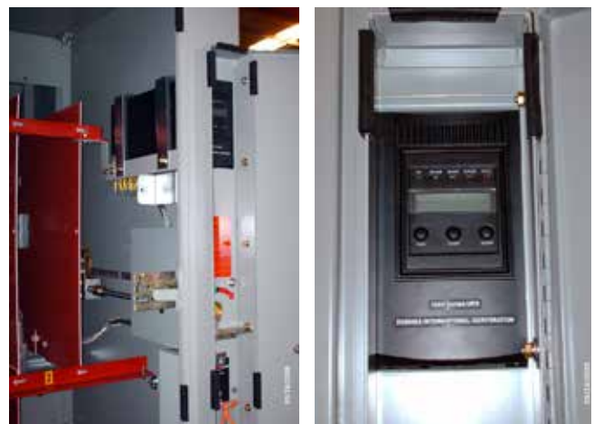
Figure 13. UPS tower-mount design installs in the enclosure stile above motor operator and extends into interior supported by a steel tray and secured by brackets. The 1.0kVA UPS unit is able to supply uninterruptable, single-phase power adequate to operate the motor operator for an extended period of up to 7 minutes at full load after control power has been lost. The unit includes a wide LCD display and also features programmable load-shed receptacles and can be provided with an optional network interface card and an optional environmental monitoring device.
