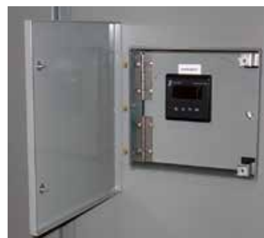
Figure 16. The digital power monitoring meter that allows real-time display of the various circuit parameters is mounted on a hinged, bolted panel in a low-voltage compartment that is isolated from high voltage.
