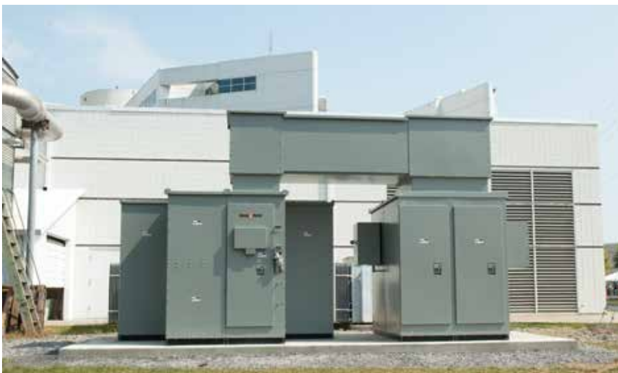
Figure 3. Automatic-transfer switchgear with Fast-Trip Transfer motor operators is pictured in the photo above. Transfer to the alternate source is achieved in approximately twenty (20) cycles.
