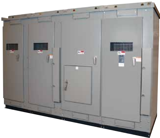
Automatic Source Transfer
