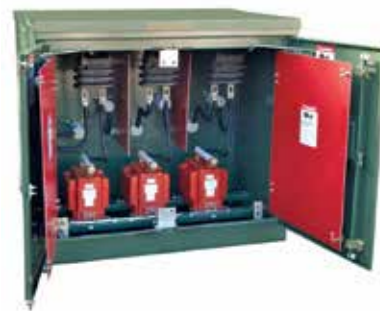
Metering Transformer Compartment With Barriers Secured Open
