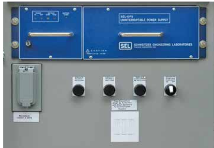
Figure 9. The Federal Pacific automatic-transfer scheme includes a UPS (at top in photo), test pushbuttons to simulate loss of source voltage and over-current lockout to allow verification of the functionality of the transfer scheme, and a duplex outlet for connection of a laptop computer.
