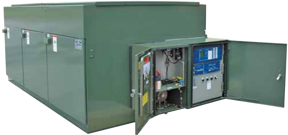
Figure 1. Exterior view of a six-compartment Federal Pacific Automatic-Transfer, Pad-Mounted Switchgear showing the motor operator and control compartment on each side. The control compartment contains the Federal Pacific Automatic-Transfer Software Program in the SEL-451 Relay. The Federal Pacific Switch Operators are in separate compartments. The automatic transfer system provides the customer with two independent power sources to assure service continuity for critical loads. The Federal Pacific Live-Front Automatic-Transfer Pad-Mounted Switchgear is configured in a similar manner. For views of switch and fuse compartments for Federal Pacific Live-Front Pad-Mounted Switchgear refer to pages 9 and 11, and for Federal Pacific Dead-Front Pad-Mounted Switchgear refer to pages 31-33.
