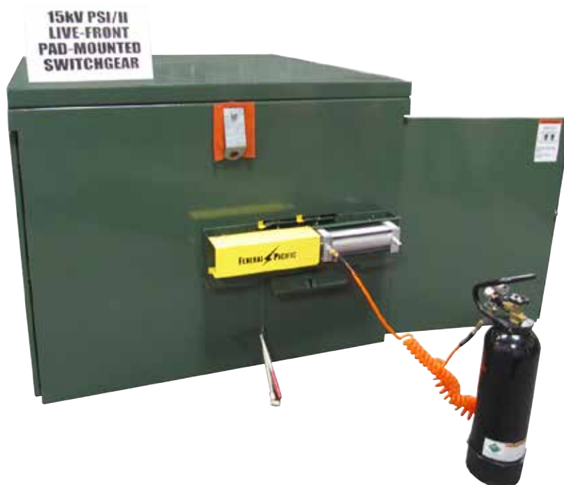
Figure 1. PROM-PM Installed on PSI/II, with Tank and Hose.
