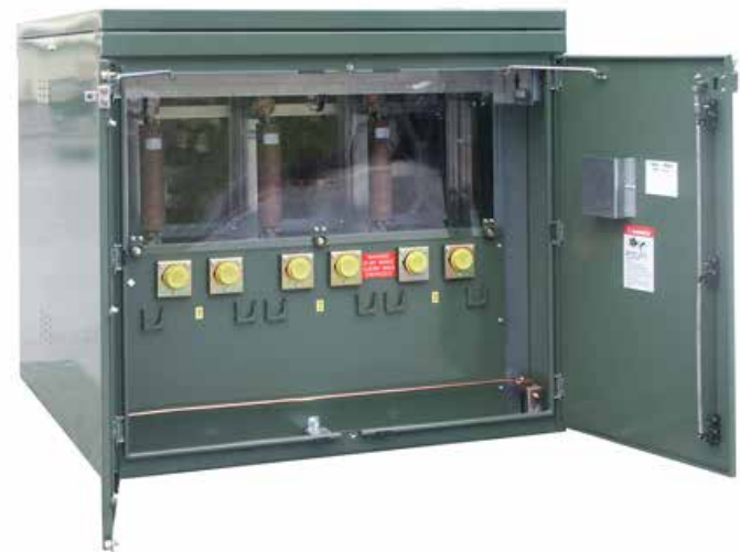
Figure 3. Incoming connections are through bushing wells that accommodate inserts and elbows (not furnished) to the protective devices, which in this installation are current-limiting fuses visible through the polycarbonate barrier.
