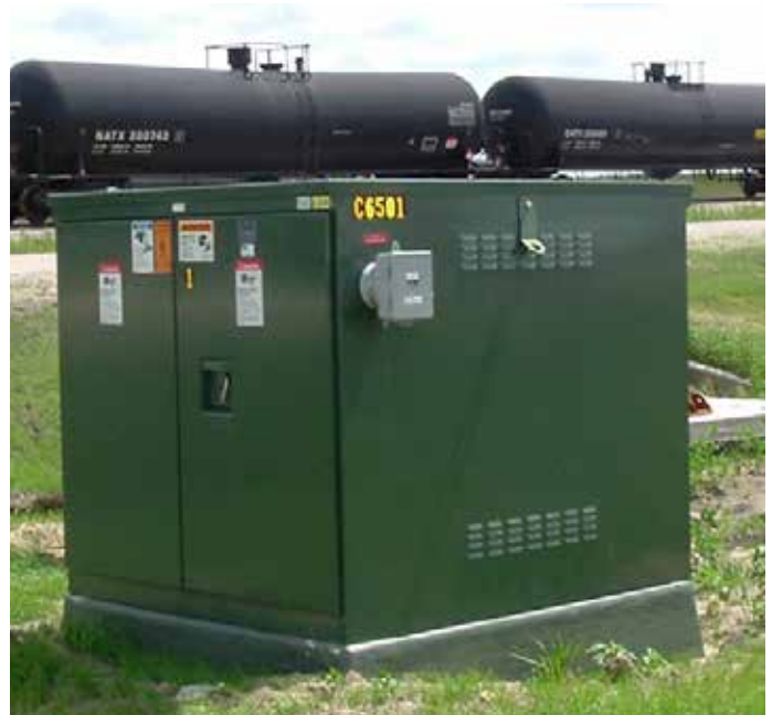
Figure 9. Pad-mounted capacitor banks provide an esthetic installation, avoiding overhead clutter.
