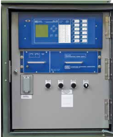
Figure 1. View of typical low-voltage control cabinet (above) that includes the automatic-transfer control relay and associated components.
