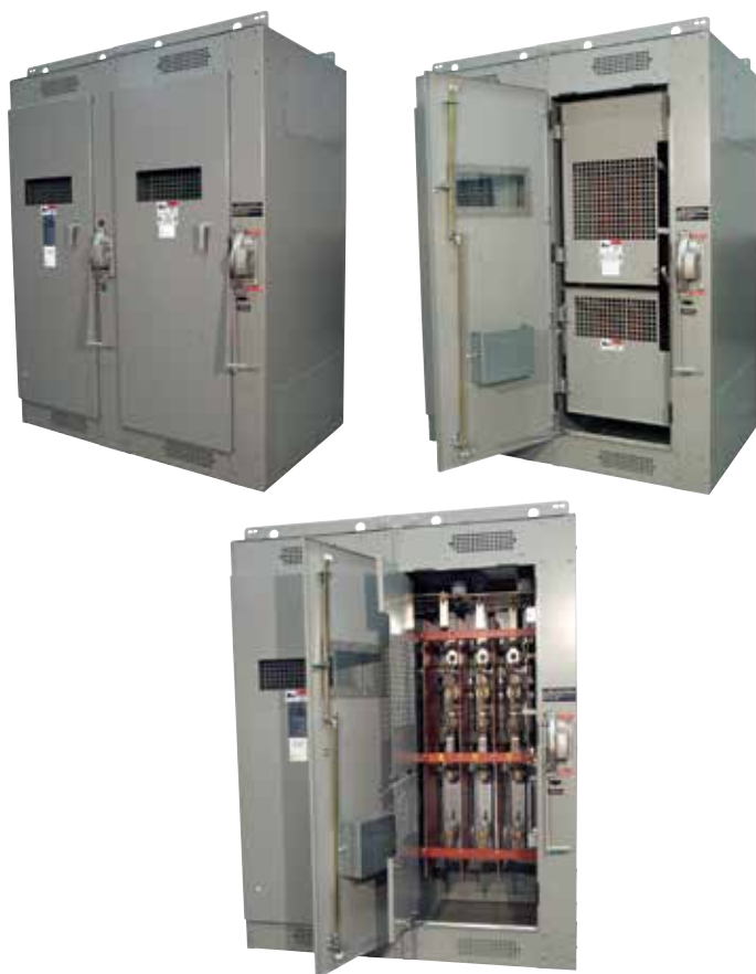
Pictured above are typical feeder bays with automatic-trip (shunt-trip) switches, providing feeder isolation when a single-phase condition (such as a blown feeder fuse) occurs.
