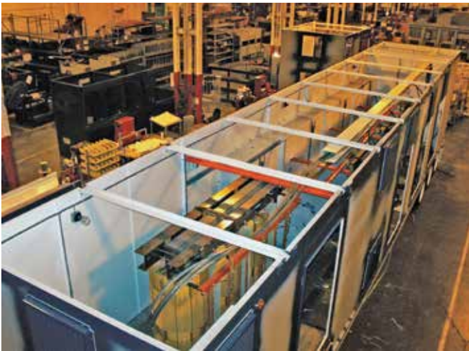
Figure 17. Portable-trailer mounted substation shown completed in Figure 18 is shown above during assembly at the factory.
