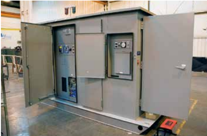
Figure 9. A skid-mounted switching station with circuit breakers and controls with easy access to the interior is pictured above.
