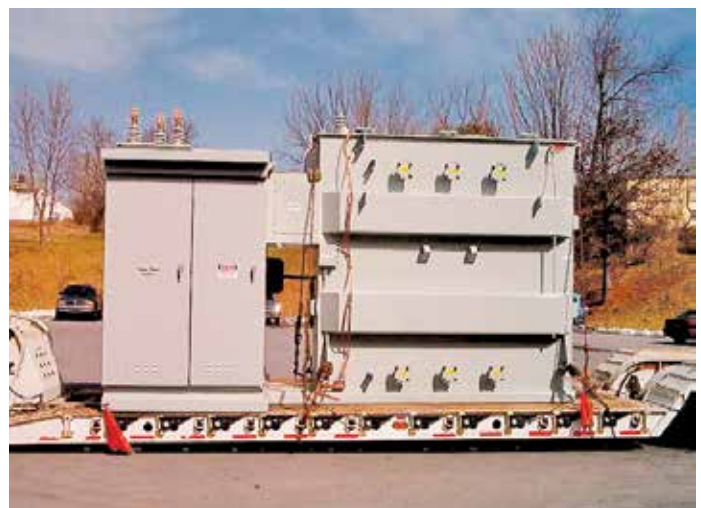
Figure 14 Portable skid-mounted substations provide immediate support for fast developing customer loads while permanent substation sighting is being negotiated and constructed.
