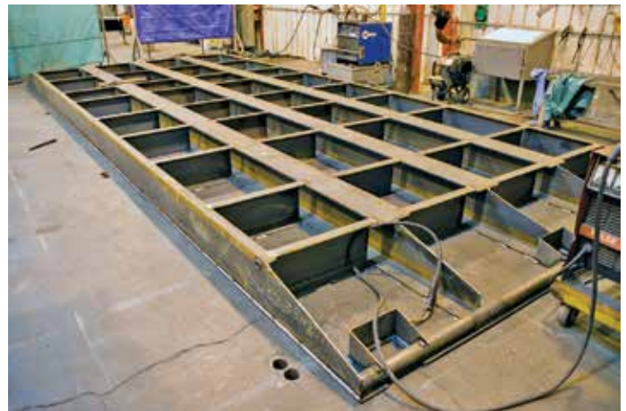
Figure 2. Fabrication, layout and welding of the heaviest gauge materials into sophisticated configurations are readily handled.
