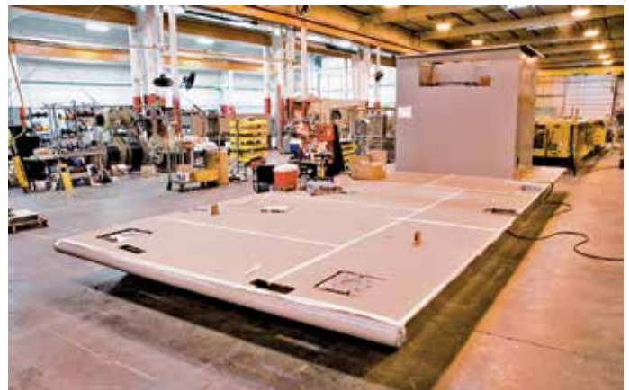
Figure 4. After painting, work surfaces are protected during installation and connection of ancillary components.
