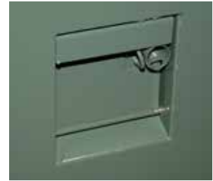
Figure 3. The door handle and door latch pocket are stainless steel. The padlock is removed, allowing access to the security bolt.
