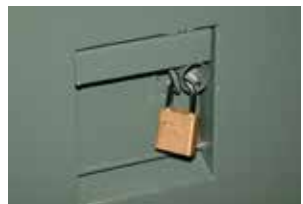
Figure 8. Always close, latch and padlock the enclosure door before leaving the unit or when working on the opposite side.
