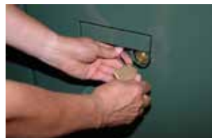
Figure 7. Padlock cannot be inserted until pentahead bolt is fully tightened.
