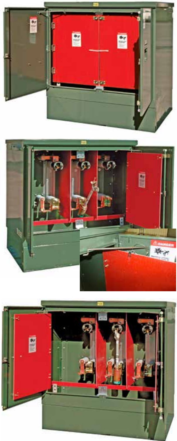
Figure 14. View of FTDF Fuse-Compartment side with external door and hinged barriers secured open. Top photo shows exterior door secured open and hinged barriers secured in place with penta-head (or optional hex-head) bolts. Center inset shows hinged barrier secured to enclosure door by inserting large cable-connected cotter pin into clip on barrier. Center photo shows fuse assembly positioned in the hinge of the fuse mounting prior to verifying proper engagement of contact rod. Bottom photo shows fuse assembly fully closed and latched.
