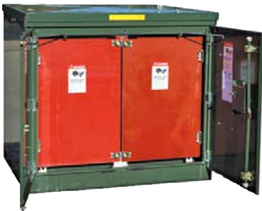
Figure 7. Open door view of PMDF with inner barriers bolted in place.
