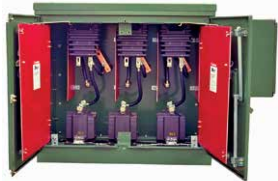
Figure 8. Open door view of metering transformers with fiberglass inner barriers secured open.
