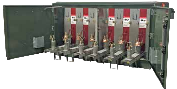
Figure 2. Open fuse panels to provide additional space to allow entry into the interior of the high-voltage compartment.
