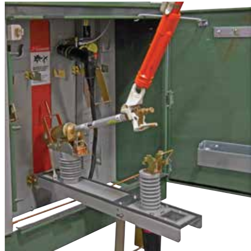
Figure 5. Shotgun clamp stick secured to fuse pull ring and fuse assembly being lifted from the latched position and being removed from fuse hinge.
