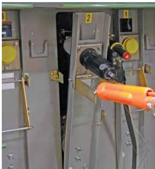
Figure 25. Fuse mounting being lowered to access fuse (or raised to reinstall fuse).
