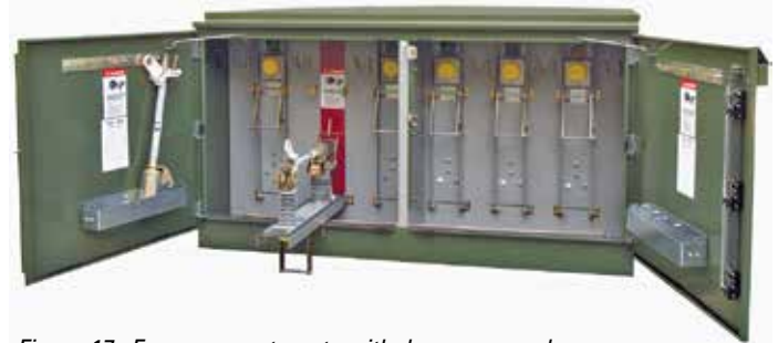
Figure 17. Fuse compartments with doors secured open.
