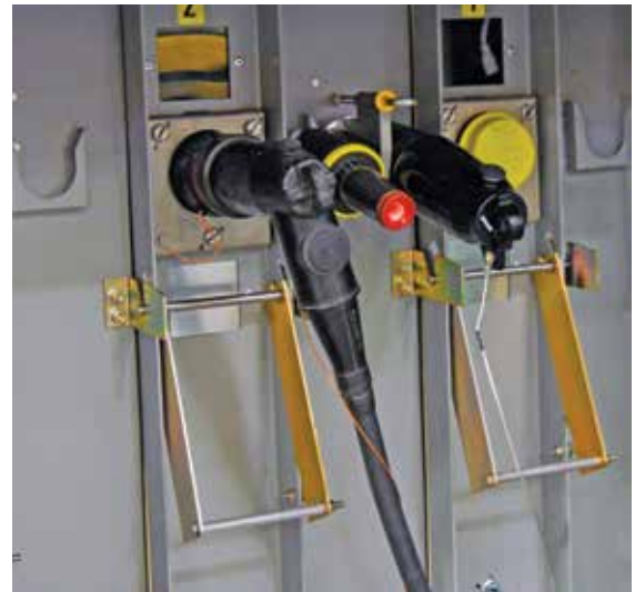
Figure 18. Feed through standoff bushing installed on parking stand.
