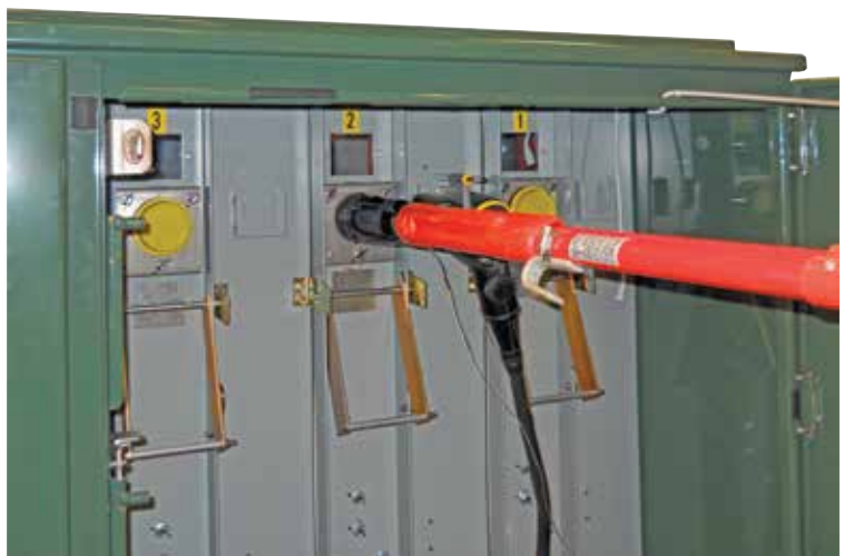
Figure 22. Insulating protective cover installed on bushing-well insert.
