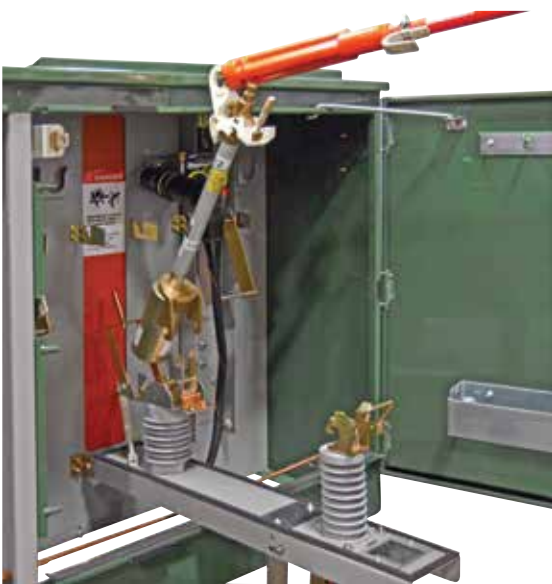
Figure 29. Shotgun clamp stick secured to fuse pull ring and fuse assembly being lifted from the latched position and being removed from fuse hinge.
