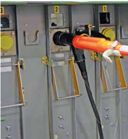
Figure 20. Shotgun clamp stick secured to elbow with elbow in process of being removed/connected to bushing insert.
