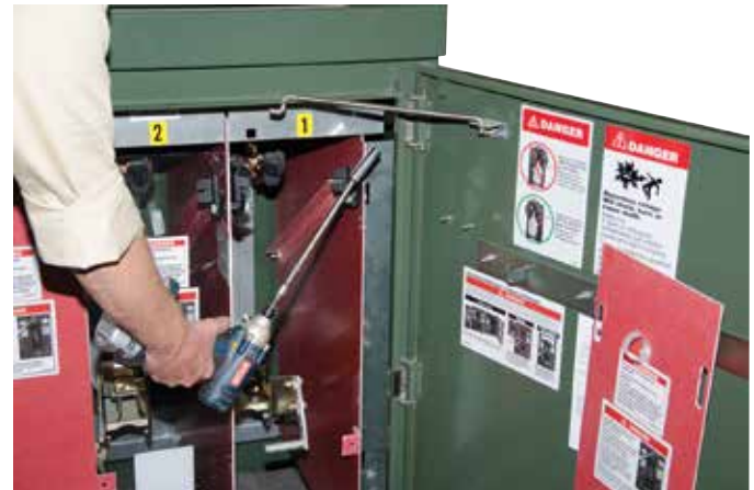
Figure 2. Preparing to remove roof retaining hardware. Note 9/16" socket on extension bar with wobble attachment and power driver.
