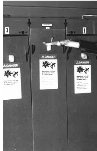
Figure 19. Lift off fuse DP barrier.
