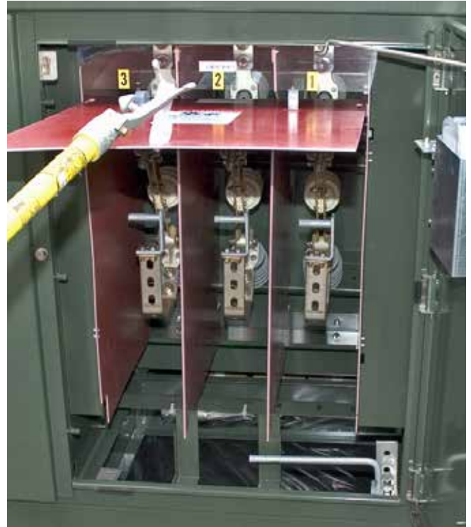
Figure 18a. Use grappler tool inserted in bottom barrier hoop and raise barrier above horizontal to slide into alternate position between switch contacts.
