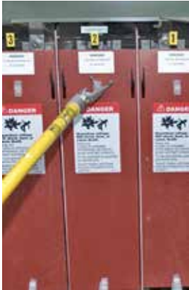
Figure 19. Lift off (or install) fuse DP barrier using long prong on grapple tool.
