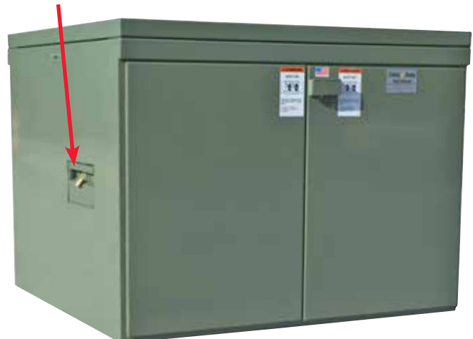
Figure 16. Exterior view showing switch operating pocket access cover.
