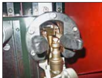
Figure 24. Adjust fuse-hinge assembly when contact rod does NOT engage latch face or latch gap exceeds 1/8".
